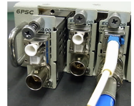
Figure.1 OE converter installation
